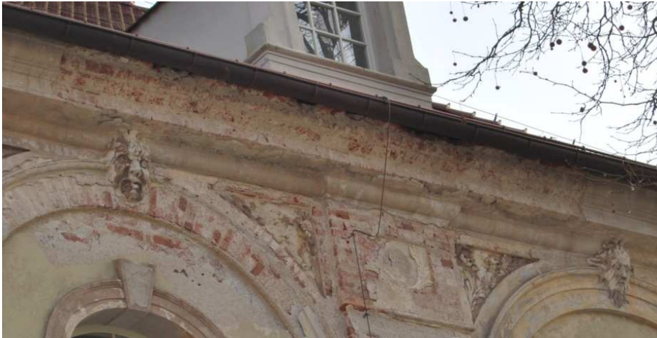
Fig. 10. Deteriorating east façade (fot. W. Sokołowski)
